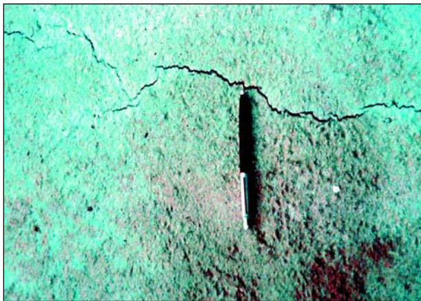
Figure 1. Plastic shrinkage cracking
