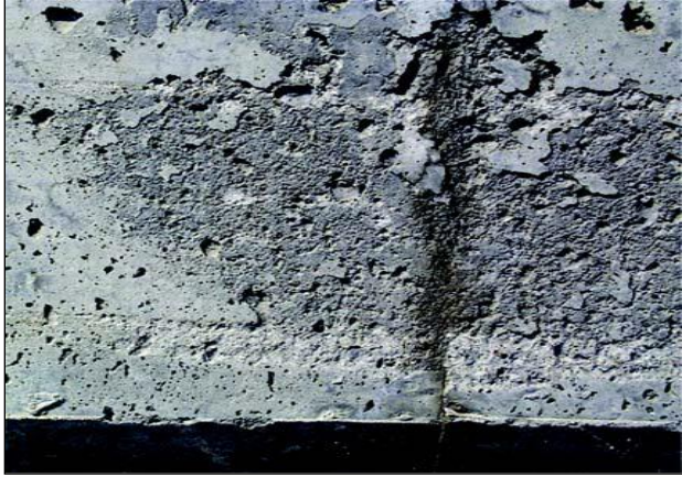
Figure 3. Scaling of concrete
